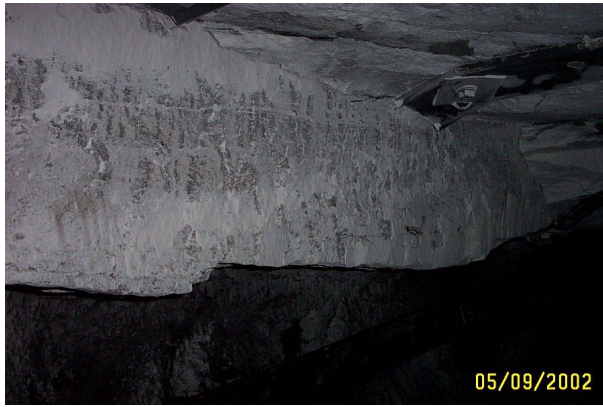
Plate 1 Vertical joint bounding roof fall that roadway to joint in Plate 1.
